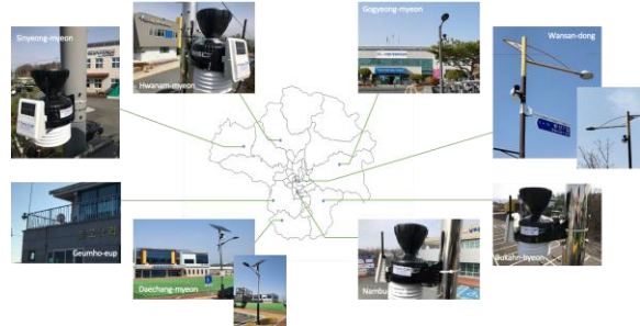
<Fig. 11> Yeongcheon-si IoT Weather Station Installation Status for Demonstration Technology Verification
